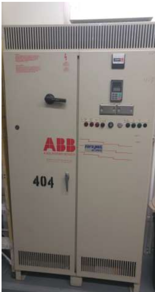
Deep Well Pump 404 Old VFD
