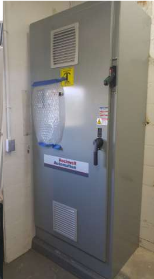
Deep Well Pump 404 New VFD
